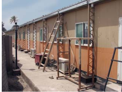
Reinforcement for collapsing building roofs at the Hilla Police Academy: another example of poor construction under a contract awarded to Bloom.
